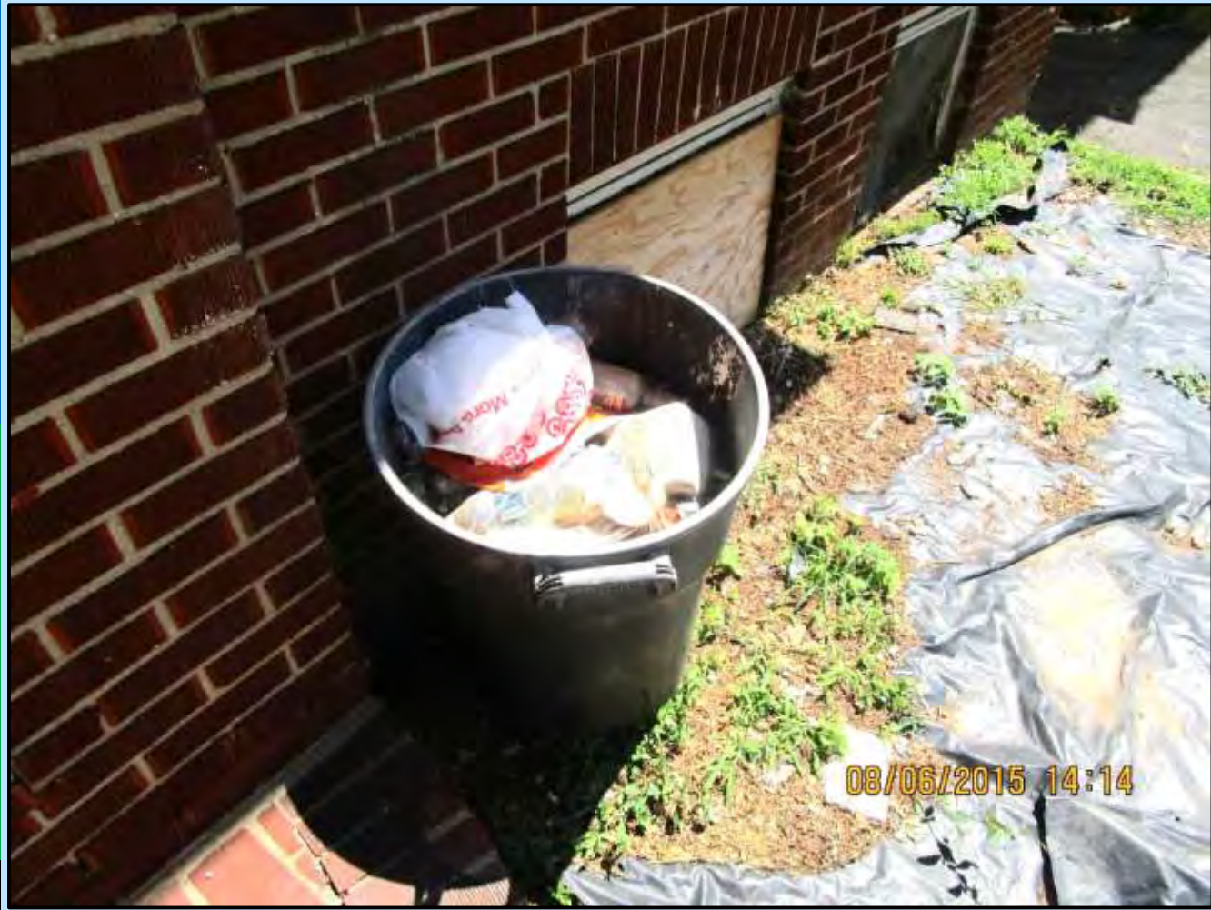
Both the back and front yards of the Bank of America foreclosure were littered with longstanding trash, unraked leaves, loose wires and other debris.
